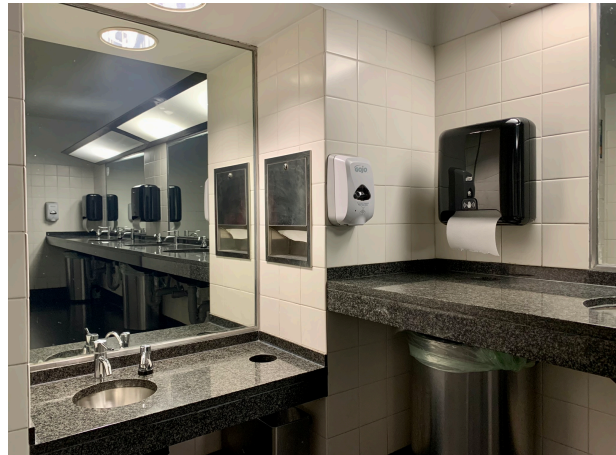
The restrooms on the first floor features both standard and accessible height sinks with motion sensor water faucets, motion sensor soap dispensers with lightly-scented foaming soap, and quiet automatic paper towel dispensers.
